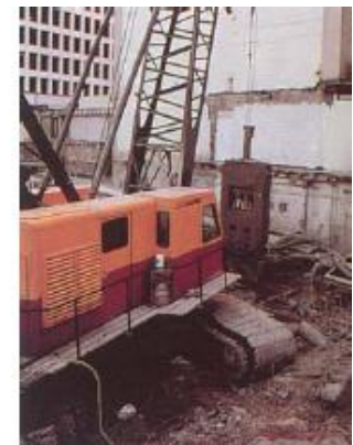
Position masts and booms
